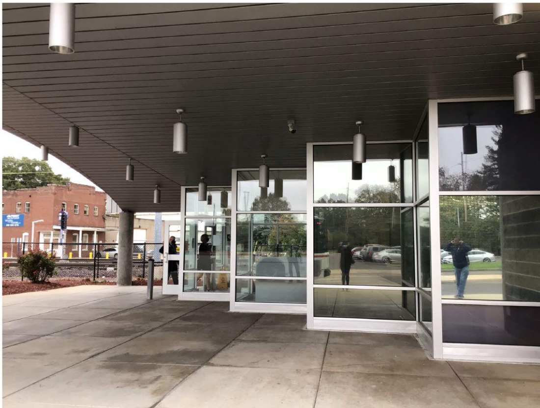
View of windows to be included as part of the project facing south.
